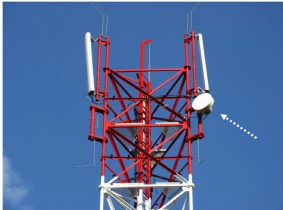
Figure 1-34 Microwave antenna at GSM site's tower
